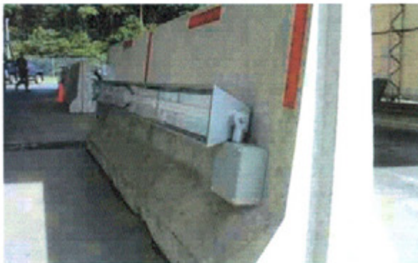
Figure 18. An example of luminaires deliberately mounted approximately 0.46 m (18 in.) A.F.G. (above finished grade), where security is a high priority. (Image provided courtesy of Magnaray International Division)
